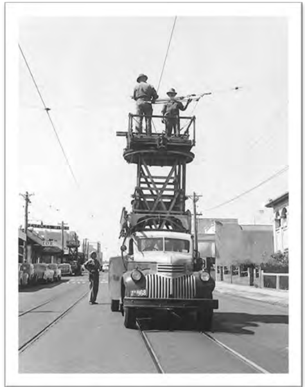
Trolley bus cables installation to replace the Mount Lawley and Inglewood tram service 1958
